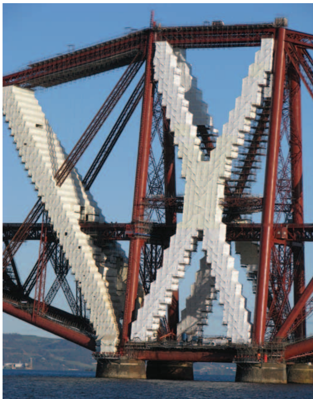
The scaffolding and encapsulation on the Forth Bridge enabled access to every square metre of the structure and ensured the safety of those working at height on the restoration project © Balfour Beatty
