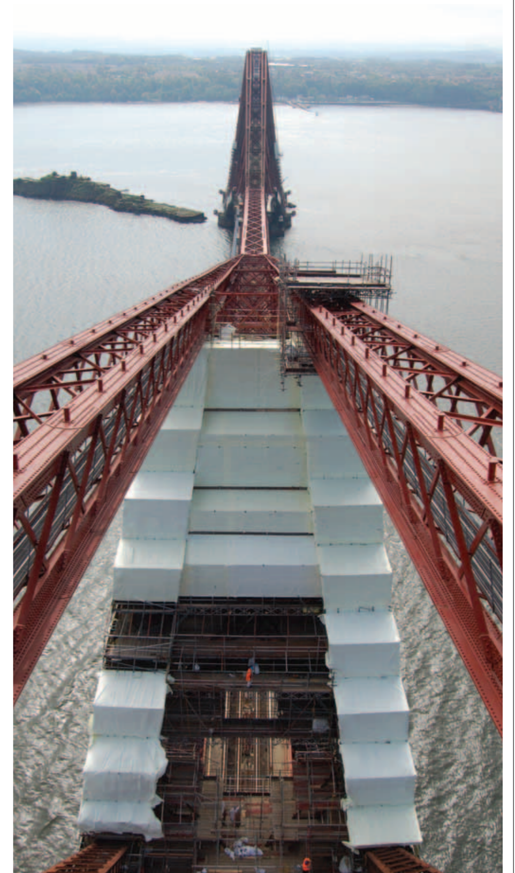
View from the top of the Fife cantilever looking south showing scaffolding and encapsulation © John Andrew
